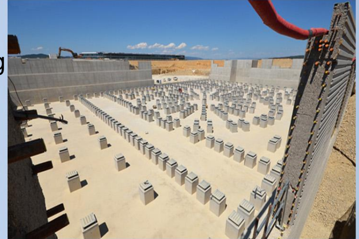
The seismic pit of the Tokamak Complex is part of the common foundation for the Tokamak, Tritium and Diagnostic Buildings. Photo: ITER Organization
