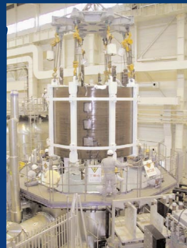
Outer module, manufactured by Toshiba, being placed outside the inner module, which has already been installed in the vacuum chamber.
