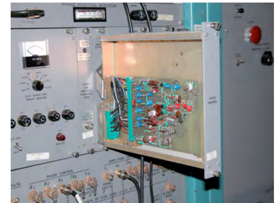
Antiquated control system to be replaced by a modern EPICS system in LANSCE-R
