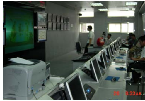
8 Control & Data system
