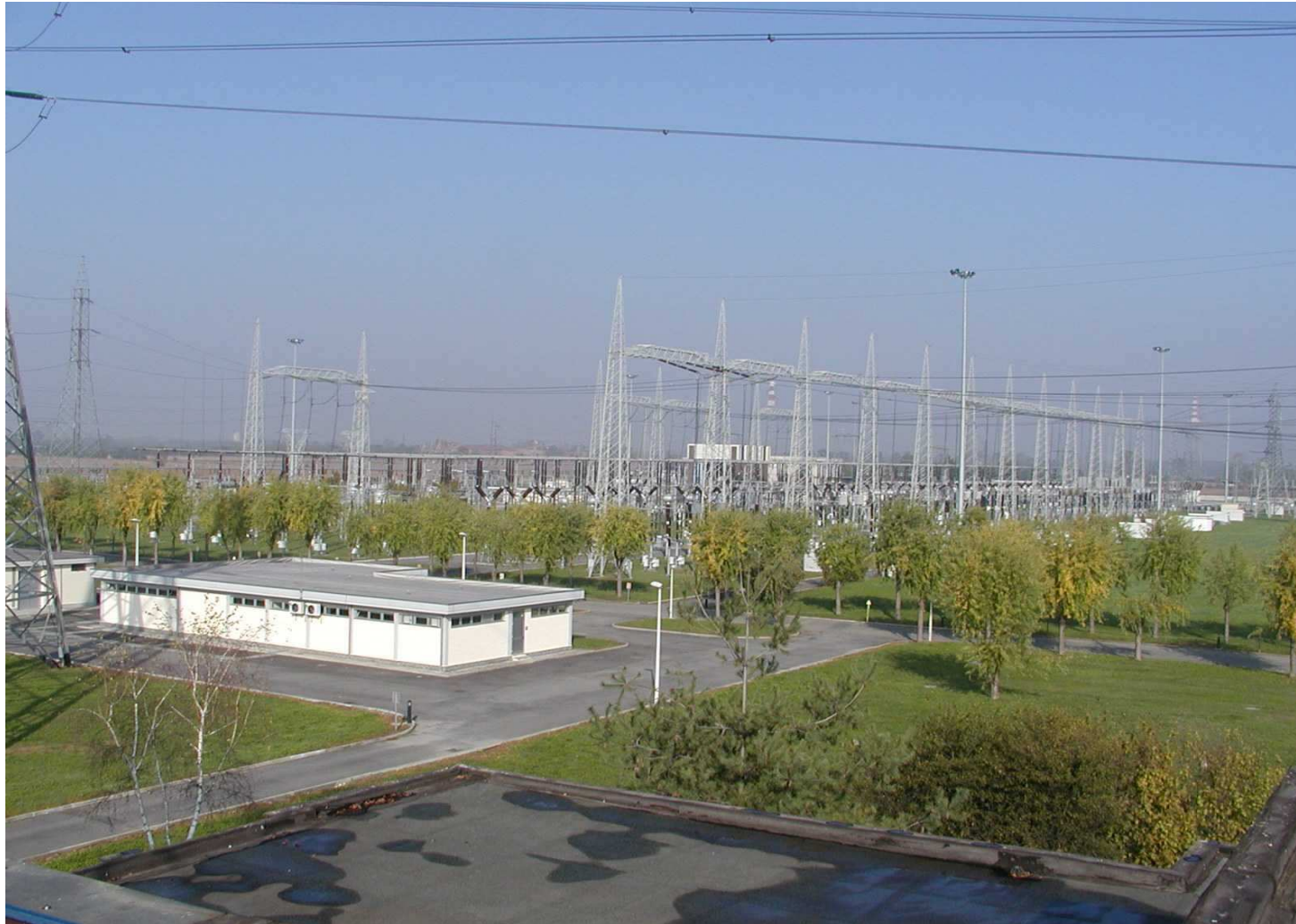
ENEL Center of Rondissone (courtesy of ENEL)
