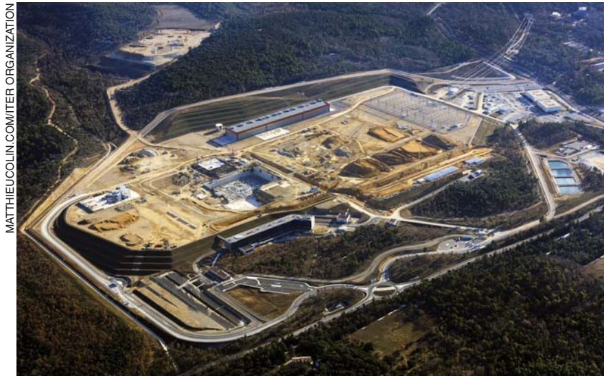
An aerial photo of the ITER complex under construction in Cadarache, France, in February 2013.
