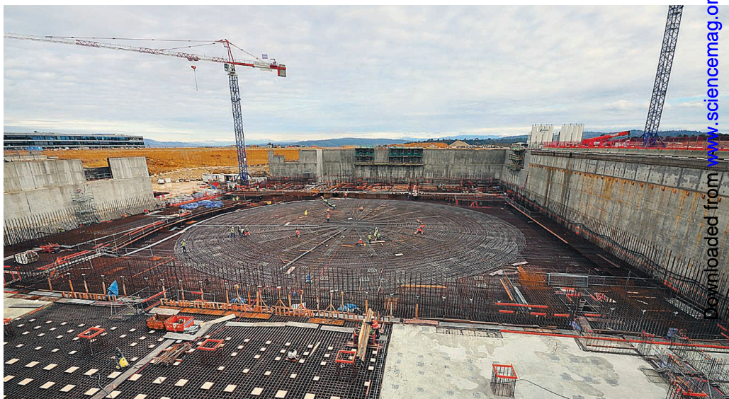
Rock bottom. Work on the circular foundations for the ITER fusion reactor was halted last June following disputes over the design. Construction did not begin again for 8 months.
