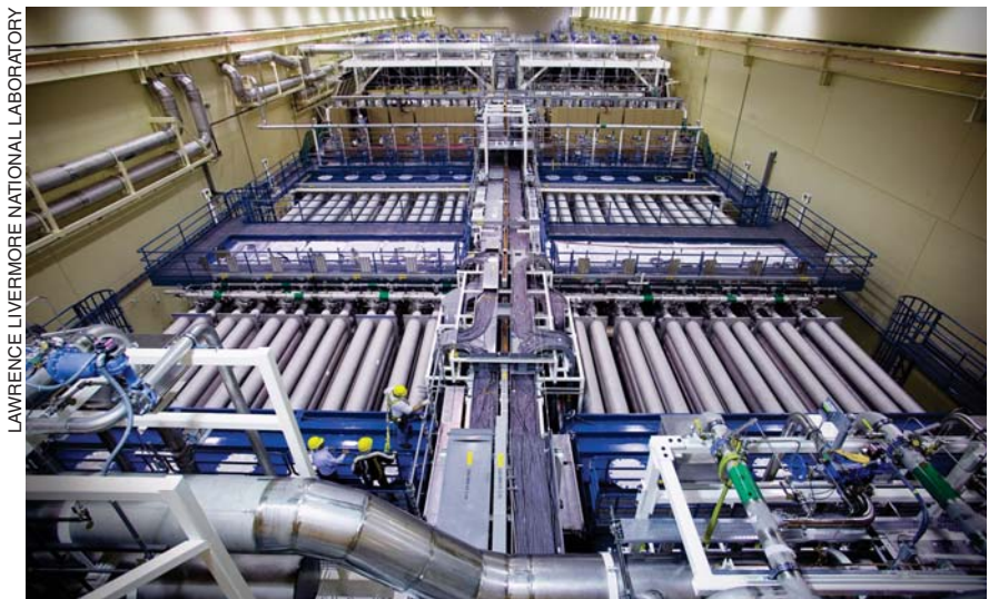
Seen from above, each of the National Ignition Facility's two identical laser bays has two clusters of 48 beamlines, one on either side of the utility spine running down the middle of the bay.
